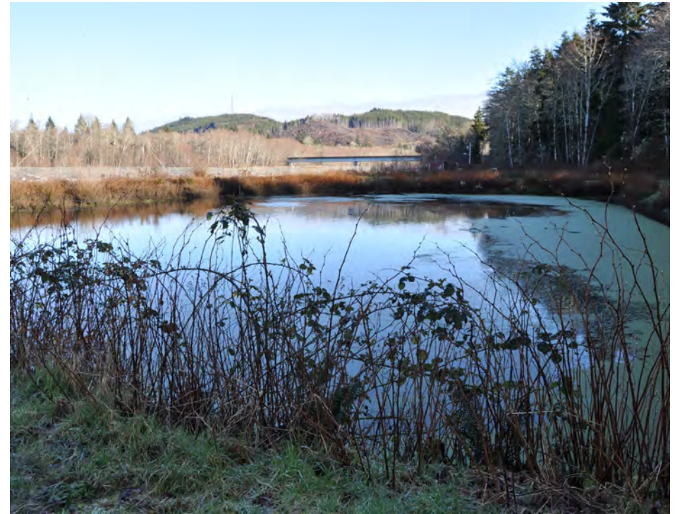
Figure 28. The "Rose Bowl," Queets' wastewater treatment facility.
