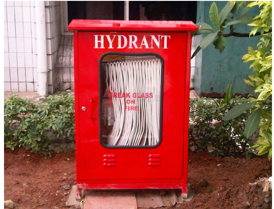
Figure 39. Fire Hose Cabinet.
