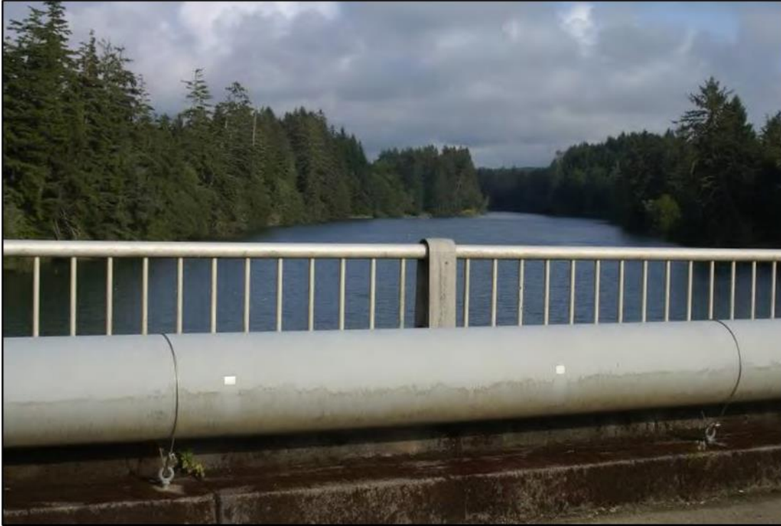
Figure 3-8 Taholah/Quinault River Bridge Water Supply Pipe
