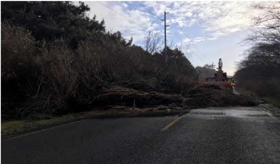
Figure 9-6 December 18, 2018 Mudslide at MP 33.5
