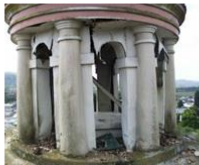
Figure 7-11 1999 Earthquake Courthouse Damage
