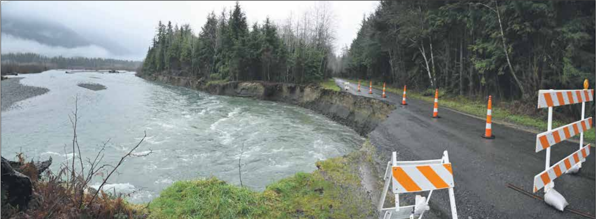
The Quinault River experienced a high flow throughout the month of December with a section of the river directly hitting the bank and creating a whirlpool effect that eroded the South Shore Road around mile 10. This area, located less than half a mile upstream from QIN's Alder River Rehabilitation site in Jefferson County, has been plagued with washout issues for decades. The road was relocated further from the river several years ago, but ongoing erosion is once again threatening the road. The road was closed before the end 2024 at the Grays Harbor/Jefferson County line. Due to the closure of the Upper Quinault River Bridge, the East Fork of the Quinault River remains only accessible by foot. Photo by Larry Workman
